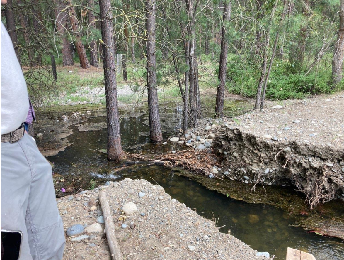
Figure 2. This photo was taken by Elizabeth Torrey, WDFW, on August 9, 2022 from approximately the same location as Figure 1. Water is still flowing through the breach toward the Yakima River Campground property. Electrical boxes for RV sites can be seen through the trees in this image.
